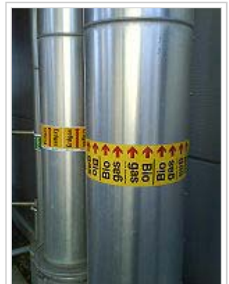
Pipes carrying biogas
